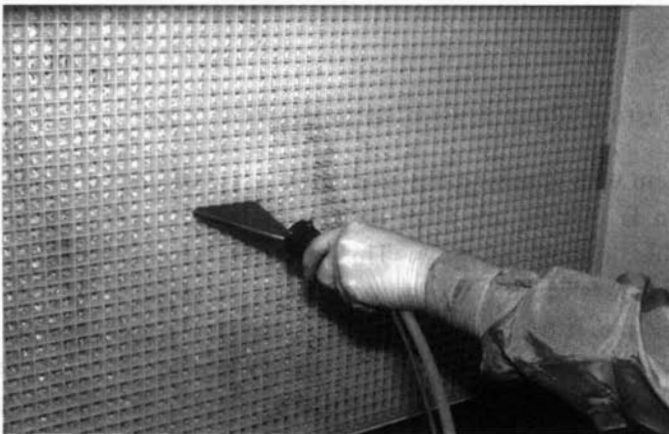
Figure 12.7 Scanning a filter azar nasim AIR CONDITIONING COMPANY
