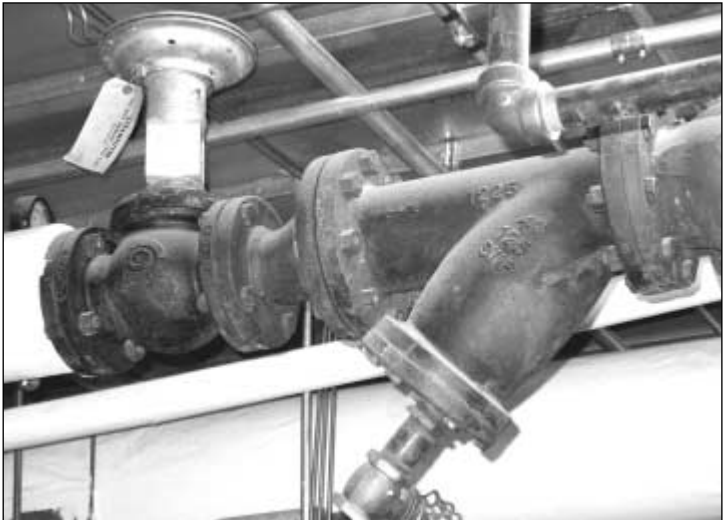
FIGURE 12.4 Steam valve and strainer.
