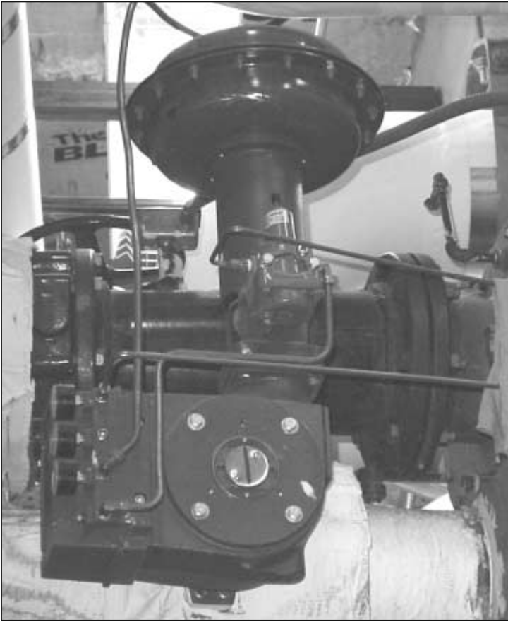
FIGURE 6.15 Five inch ball valve used in steam service.
