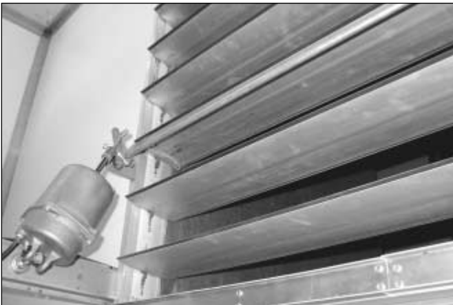
FIGURE 13.5 Pneumatic actuator on tight-seal outdoor air dampers.
