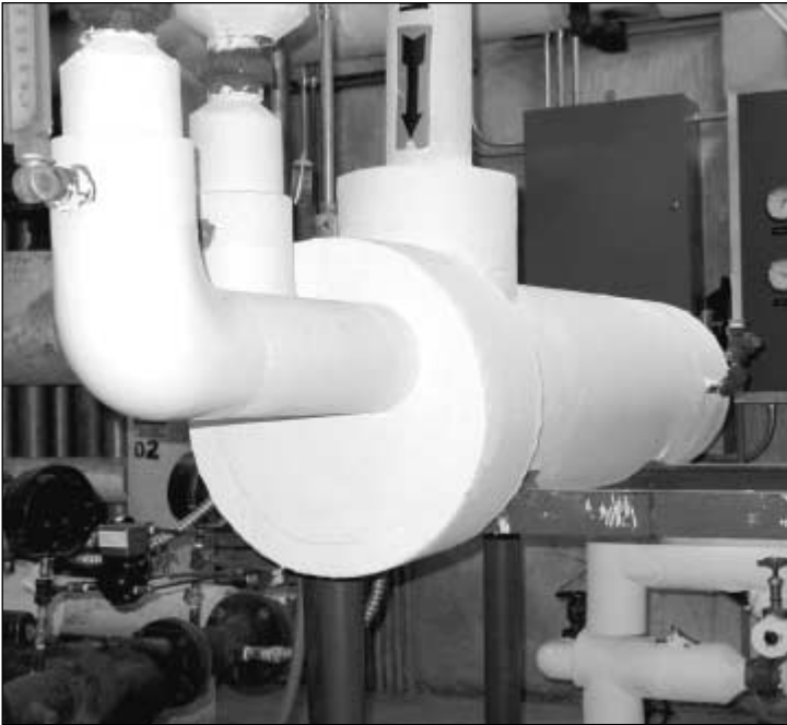
FIGURE 12.11 Insulation on steam-to-hot water converter.
