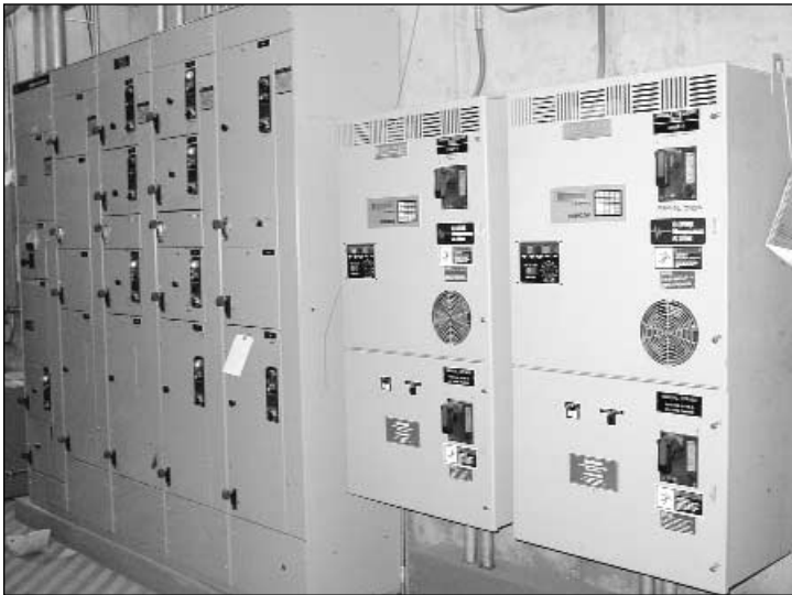
FIGURE 4.13 Motor control center (cabinet on left) and variable frequency drives (two boxes on right).
