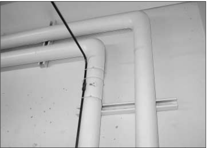
FIGURE 3.2 Insulated pipe mounted on wall brackets.
