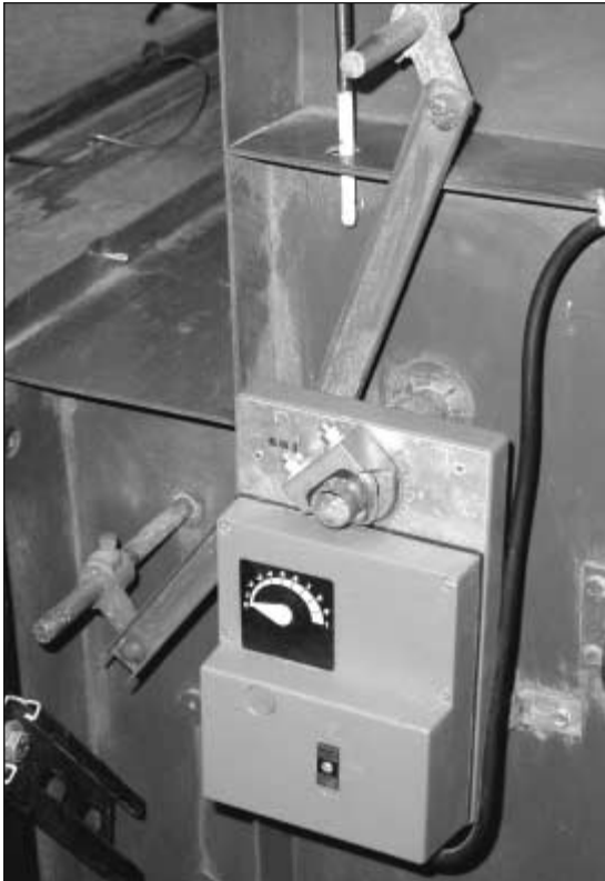
FIGURE 5.41 Electronic damper actuator and linkage.
