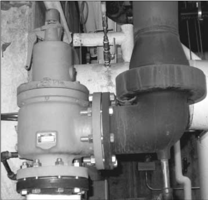
FIGURE 12.3 Steam pop-off valve (rated at 30 psi).
