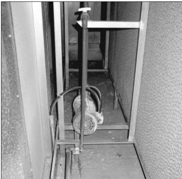
FIGURE 17.4 Swamp cooler circulation pump situated above sump.
