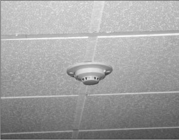
FIGURE 16.16 Smoke detector located on suspended ceiling.
