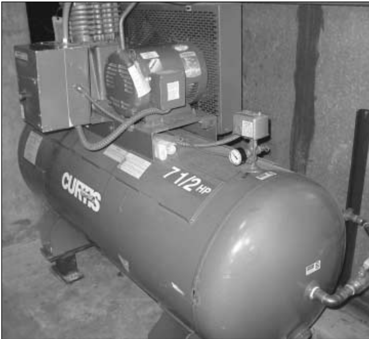
FIGURE 2.14 Combined air compressor and storage tank.
