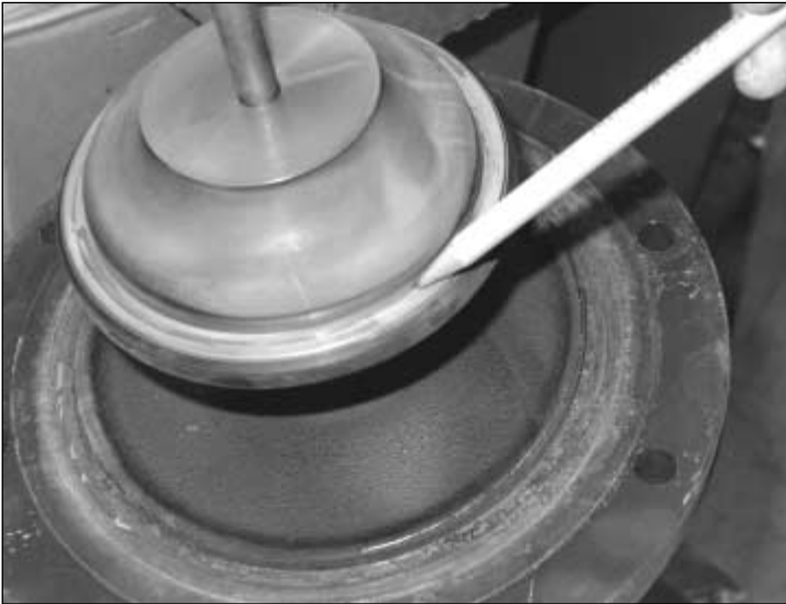
FIGURE 12.22 Valve plug on six inch steam valve.
