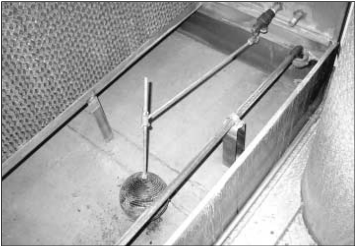
FIGURE 17.9 Swamp cooler sump refill level float not working (no water in pan).
