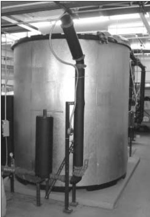
FIGURE 10.6 150 ton-hour ice thermal storage tank.
