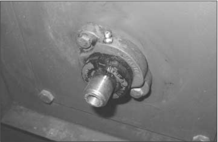
FIGURE 14.23 Fan bearing grease port on side of AHU.
