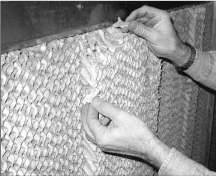
FIGURE 17.10 Old evaporative media crumbles at the slightest touch.
