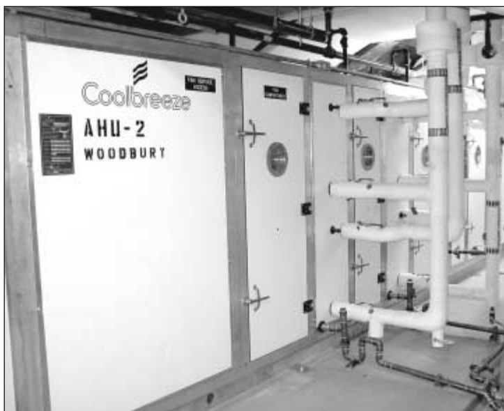
FIGURE 14.7 Large air-handling unit showing access doors.
