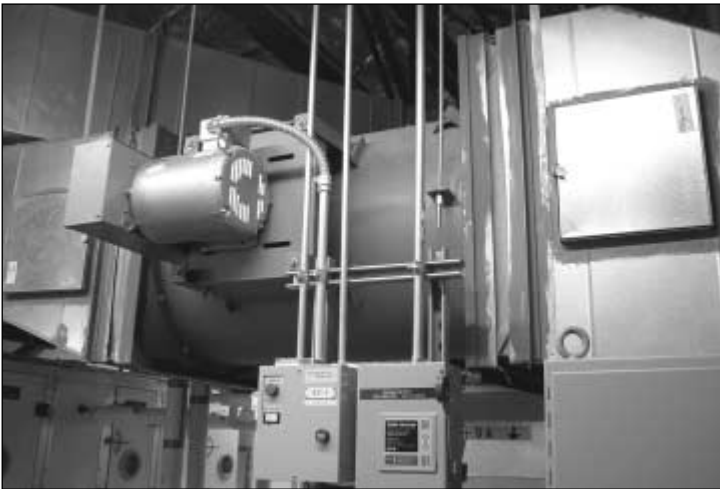
FIGURE 15.3 Return fan showing upstream and downstream duct access doors.
