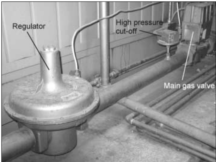
FIGURE 11.8 Boiler gas valve and high pressure cut-out.
