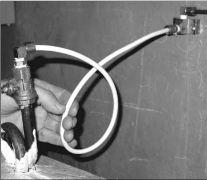
FIGURE 12.17 Transmitting steam pressure signal with Teflon tubing.
