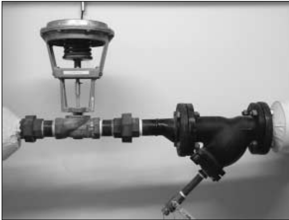
FIGURE 7.19 Strainer upstream of hot water valve.
