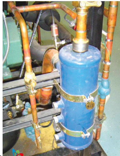
Figure 10–5 Oil separator mounted on the end of the compressor rack. Photo by Dick Wirz.
