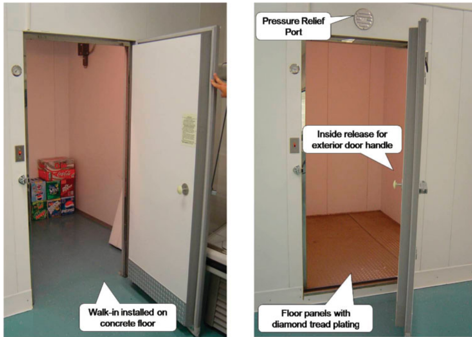
Figure 11–4 Walk-in without floor panels (left) and walk-in floor panels with diamond tread plating (right). Photos by Dick Wirz.
