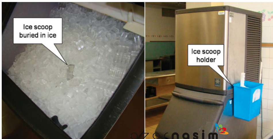
Figure 13–3 Ice scoops must be stored outside the ice bin. Photos by Dick Wirz.
