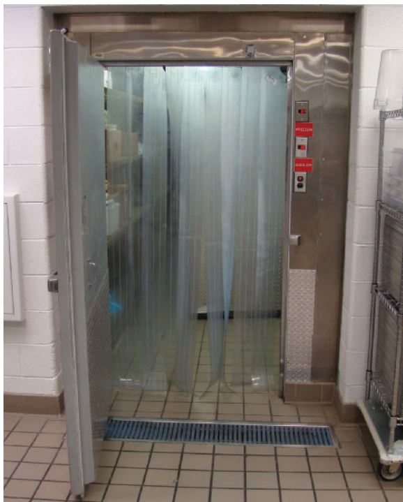
Figure 11–27 Walk-in door with strip curtains. Photo by Dick Wirz.
